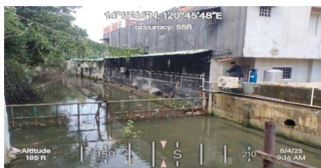
Figure 6 and 7. The (a) Design and (b) Actual photo of the Gate-typed Trash Trap installed in Brgy. Bucana Sasahan, Naic, Cavite.
